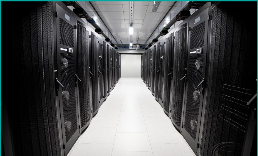
Data center aisle inside N01 Campus.
